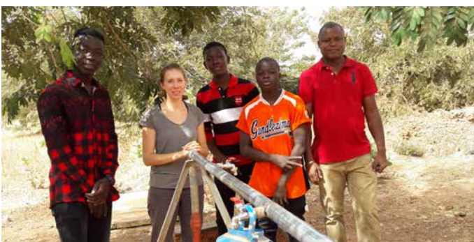
Students from Dedougou visiting the works with Véronique, member of Solidarité Saint-Gabriel
